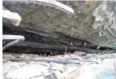
(b) Concrete in the collapse region
