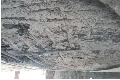
(a) Deformation of the reinforcing bar
