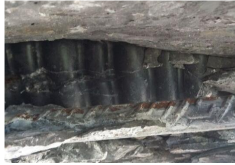
(b) Deflection of corrugated pipe
