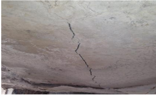
(a) Longitudinal cracks along the span direction
