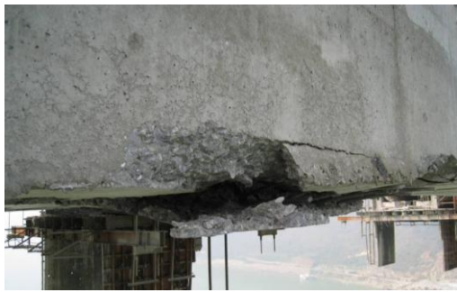
(a) Collapse of the bottom plate
