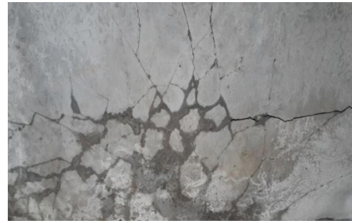
(b) Crushed zone on the bottom plate
